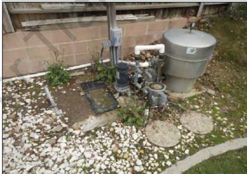
Missing pool equipment
